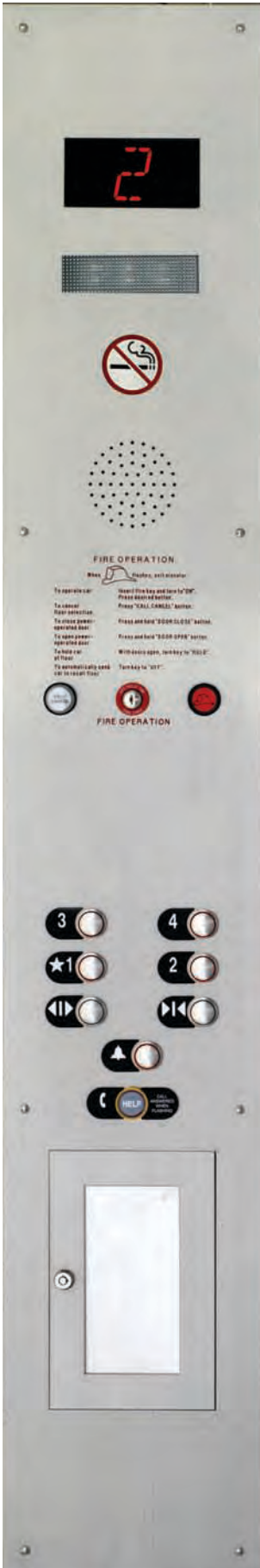
Car Operating Panel
